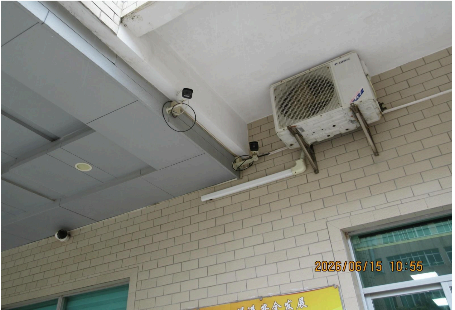
304-Loading area with CCTV camera installed.jpg
